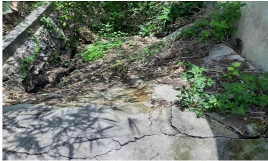
Figure 4. The point that collapsed (October 2024)
