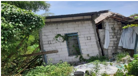
Figure 5: House Condition (October 2024)
