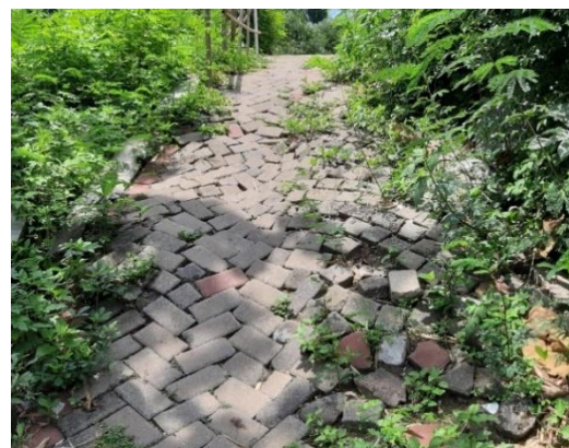
Figure 3. Road collapse (October 2024)
