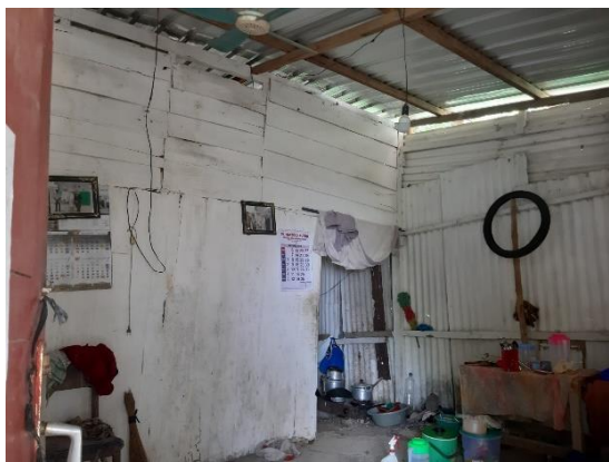
Figure 8: House Condition (October 2024)
