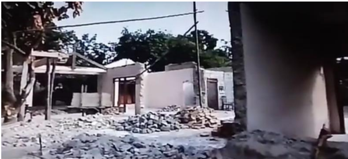
Figure 1. Building Collapsed Condition at Point K26
